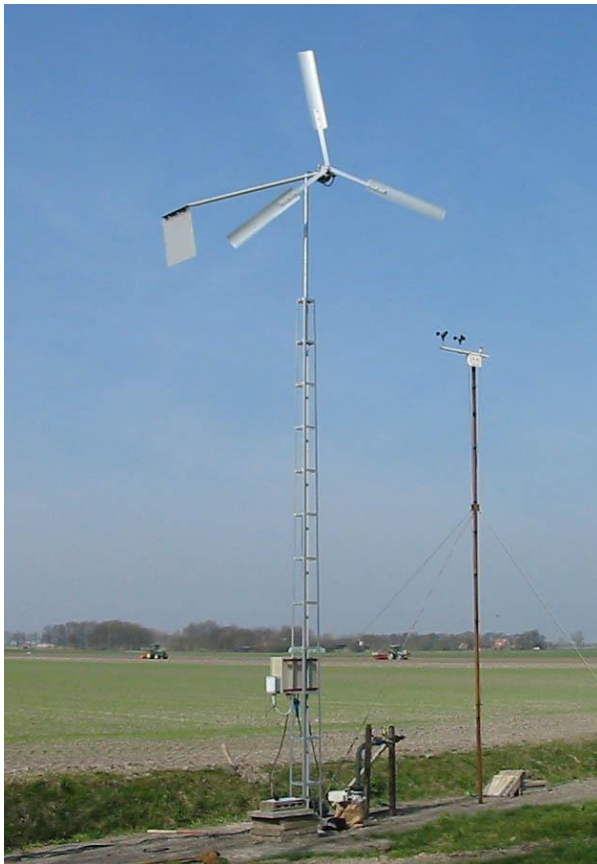
fig. 1 First VIRYA-3D prototype at the test field of Teamwork Technology in ZijdeWind
